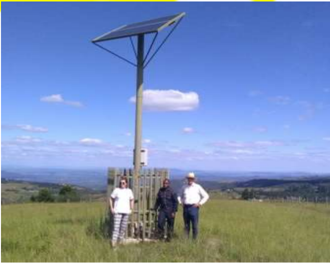
At the site of the solar borehole pump
